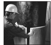
Tank & Equipment Insulation
