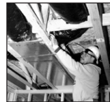
Flexible Duct Insulation
