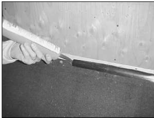
Step 1. After membrane flashing is installed, caulk along the top of curb with membrane compatible material.
