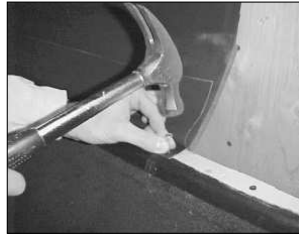
Step 2. Fold over cover membrane to expose concealed nailing strip and nail 4" oc starting 1/2" from end, using 1 3/4" roofing nails, fold cover membrane over the nailing strip.
