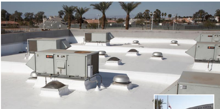
Southwest High School, El Centro, Calif. 76,000 square feet of JM PVC-60 Roofing Contractor: Roof Construction, Escondido, Calif. Owner: Central Union High School District
